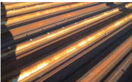
Bare Galvanize steel roof after 28 years of industrial exposure.
