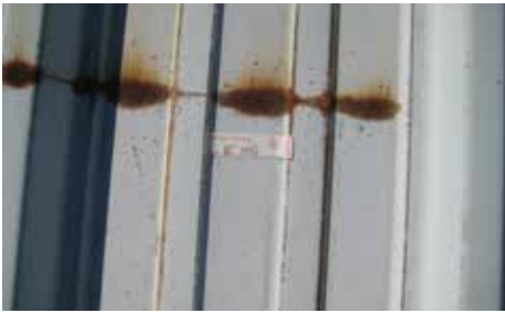
Scribe on polyester pre-painted Galvanized steel roof after 28 years of industrial exposure.
