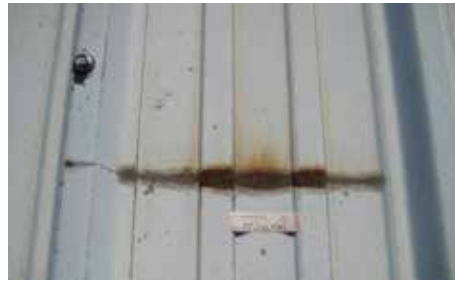
Scribe on polyester pre-painted Galfan steel roof after 28 years of industrial exposure.
