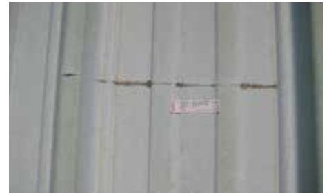
Scribe on polyester pre-painted Galvalume steel roof after 28 years of industrial exposure.
