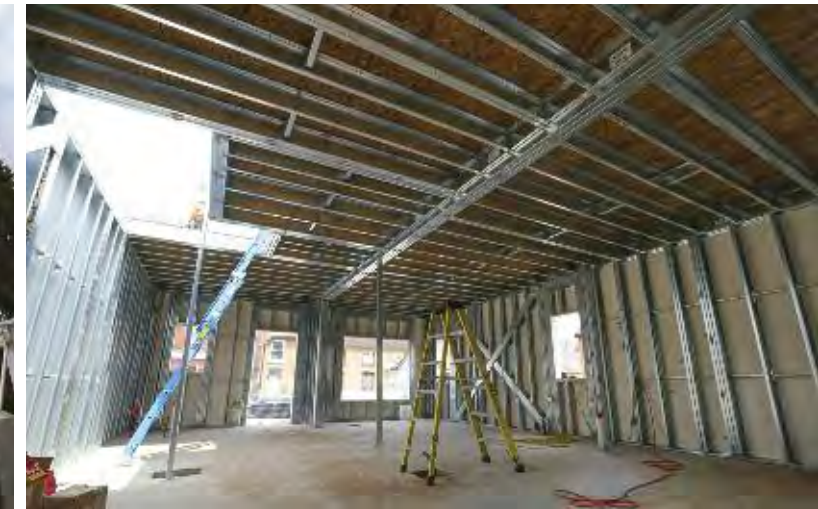
Interior view showing prefabricated roof trusses, exterior pre-assembled wall panels and interior wall studs. The floor system is comprised of a CFS panel system with a reinforced concrete overlay.
