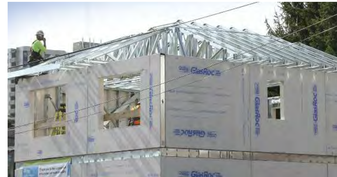
Finishing off the exterior is Stratus vertical wall cladding and AR38 Panels on the roof.
