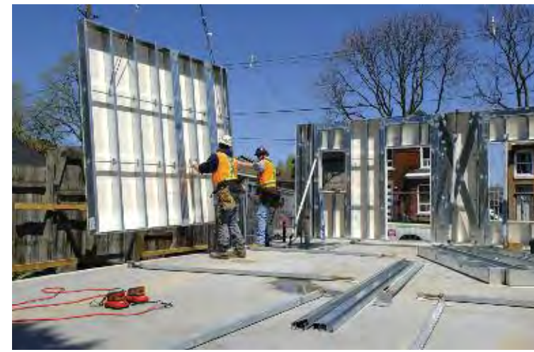
Engineered CFS wall panels are prefabricated with exceptional precision in a controlled environment, versus unpredictable field conditions. This not only guarantees a higher degree of quality, but it also prevents unexpected schedule delays due to weather conditions and other factors.
